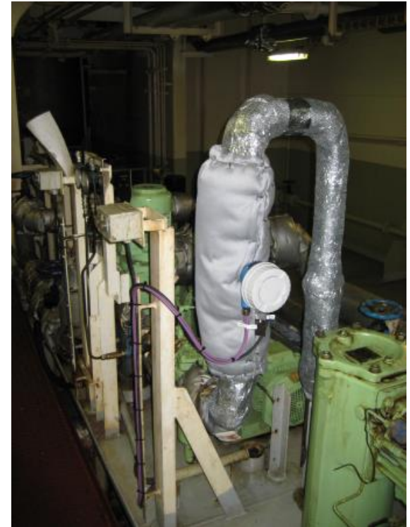
Drain Flow meter
